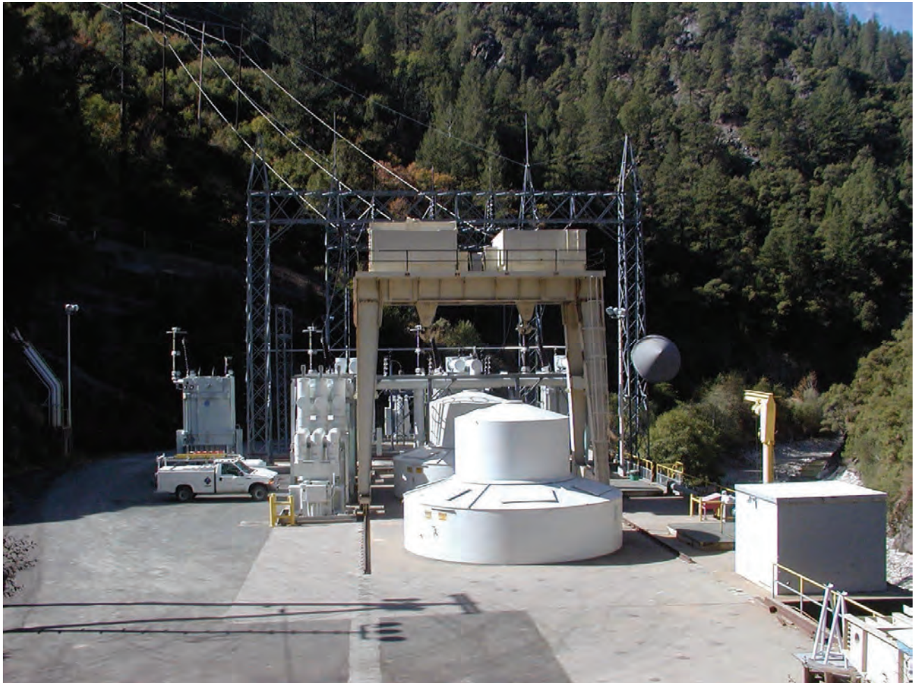
Middle Fork Power House
